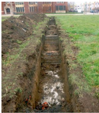
FIGURE 3. View north along Trench 3, one of the three trenches that exposed brick walls and cement basement floors.
