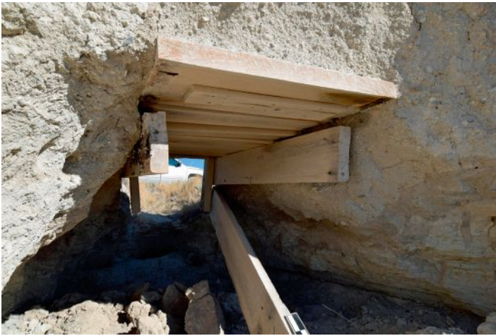
FIGURE 7. Overview of a nearly destroyed box culvert with separate strut.
