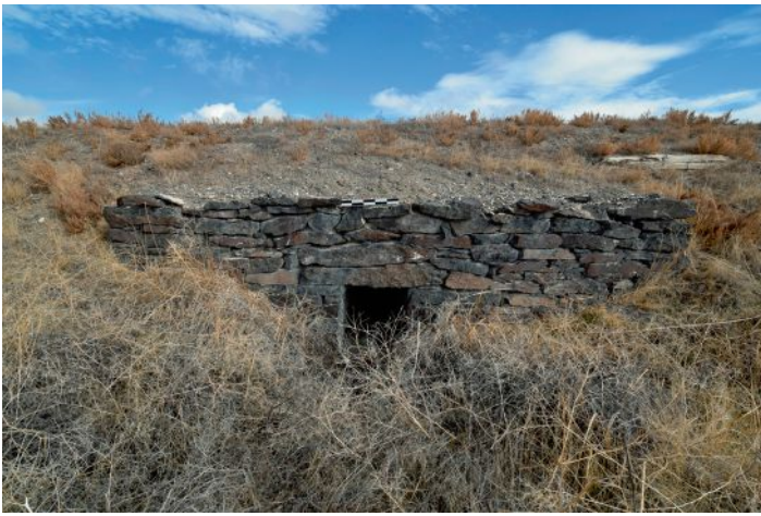
FIGURE 4. Feature 117 exceeds the other stone box culverts in terms of its complexity and workmanship.
