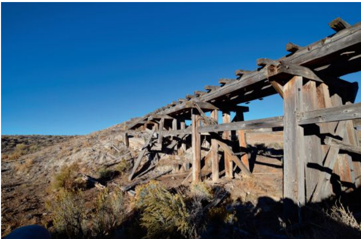
FIGURE 3. Multi-stringer trestle with five bents and girts. Note that many of the railroad ties are no longer in place on the deck.
