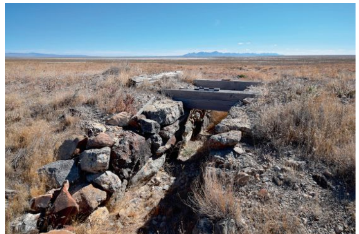
FIGURE 10. Example of a stone open-deck culvert with intact stringers that has been subjected to erosion.
