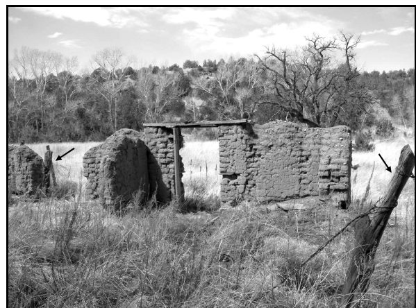
Figure 17 – East segment of front wall – back view (arrows point to fence posts)
