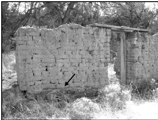
Figure 16 – East segment of front wall – front view (arrow points to rock foundation)
