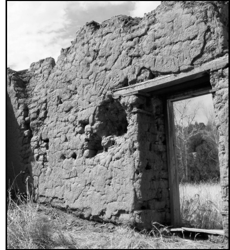
Figure 24 – Note lack of beams or other upper floor evidence between the lower window (right) and the single board remaining of the upper window sill (upper center)
