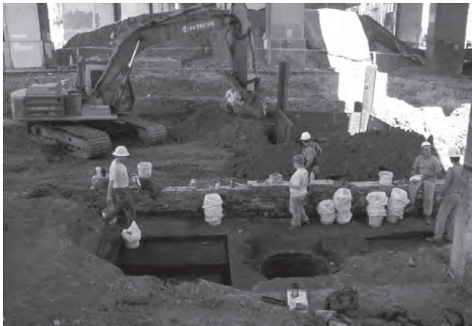
Excavation of the shell midden which is cut by a brick-lined well. The tracked excavator in the background is placing slide-rail shoring around another well.
