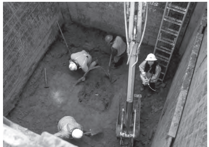
Crew working on a well inside the slide-rail shoring box on Block 10.
